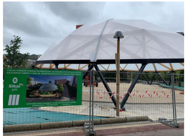
Figure 42: Construction for a New Children's Playground in Doña Casilda Park Financed by Bilbao Garbi —City Maintenance Company (Source: Nikolovski)
