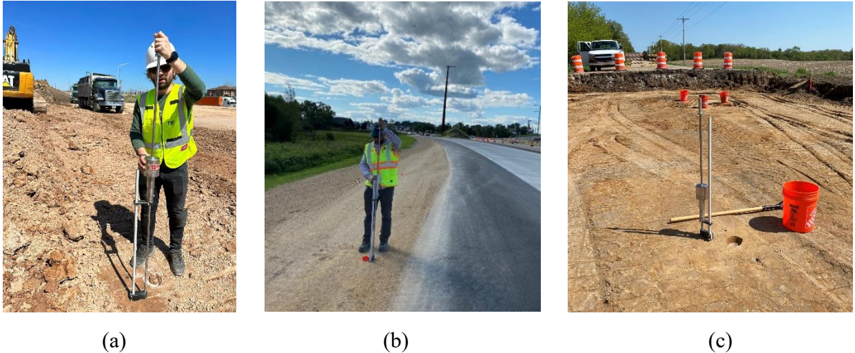
Figure 3.7 Dynamic cone penetrometer (DCP) test performed at (a) Milwaukee County, (b) Juneau County and (c) Racine County
