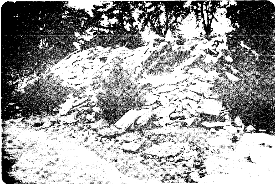
Figure 30. Broken concrete slabs armoring the bluff slope in the South \frac{1}{2} / Section 8 / T2N,R23E, Kenosha County, Wisconsin. This photo was taken on July 30, 1978.
