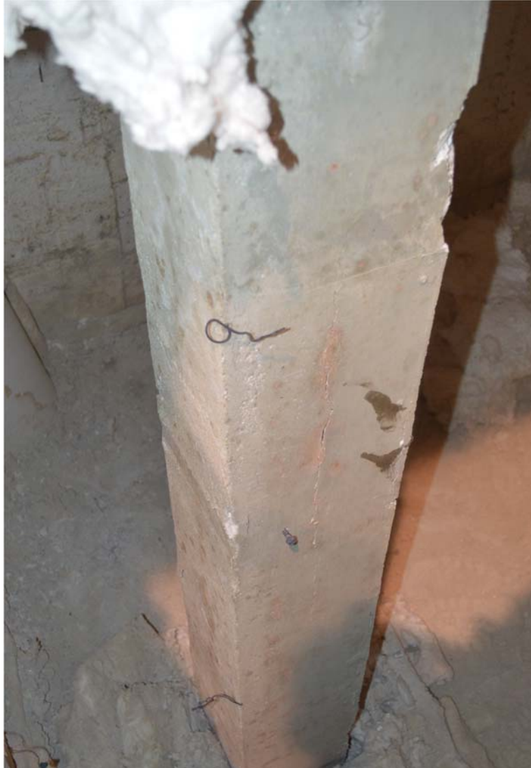
Figure 3.18. Column C-2, 40 Hours after Fire Exposure.
