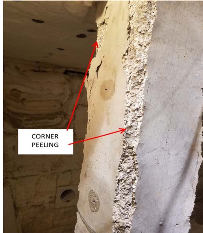
Figure 3.16. Corner Peeling of Column C-1, 40 Hours after Fire Exposure.
