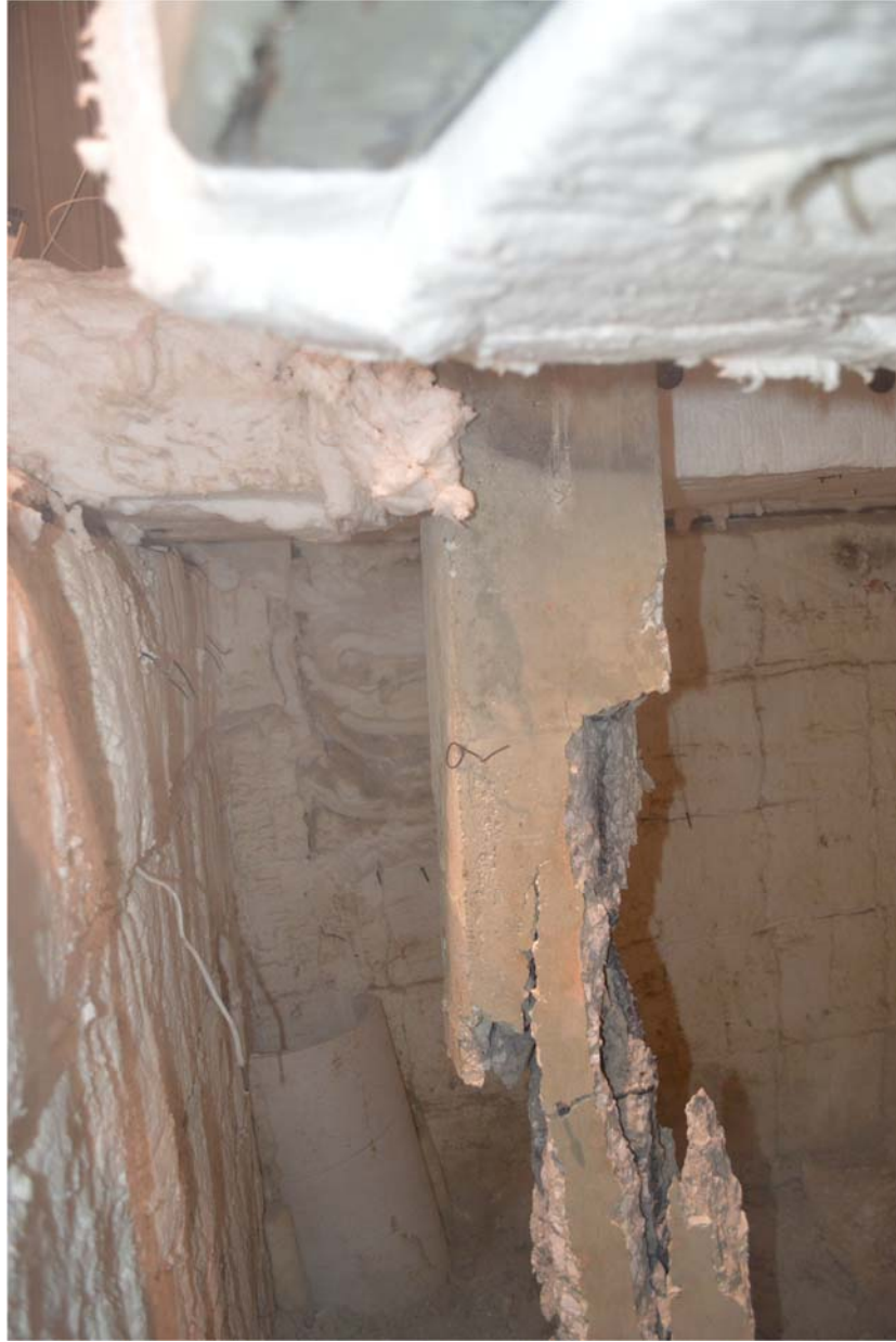
Figure 3.27. Condition of Column C-2, Post Residual Testing.
