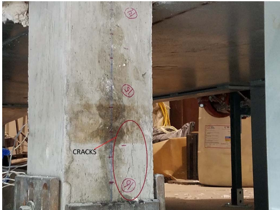
Figure 3.17. Vertical cracking at Bottom of Column C-1 During Fire Exposure; Approximately 80 Minutes into Exposure.
