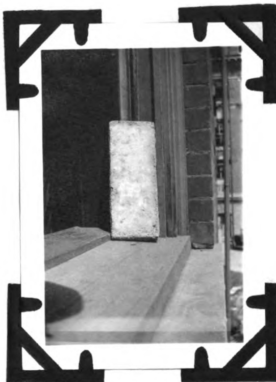
a piece of the base coat. note the porosity.
