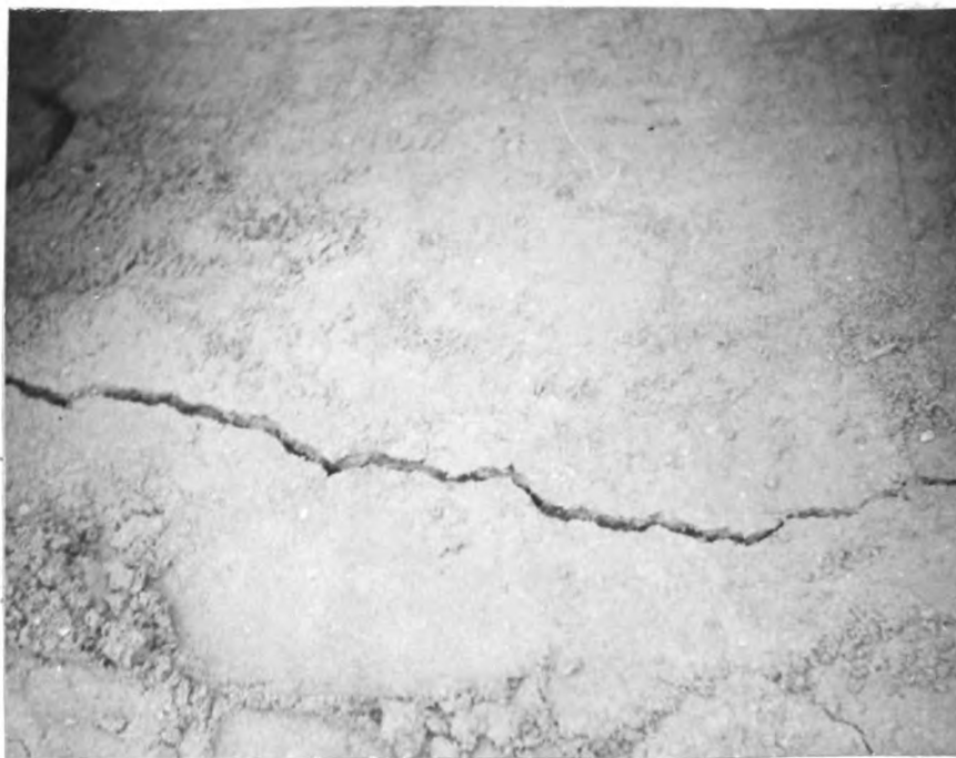
Figure 10. Ground failure caused by log.
