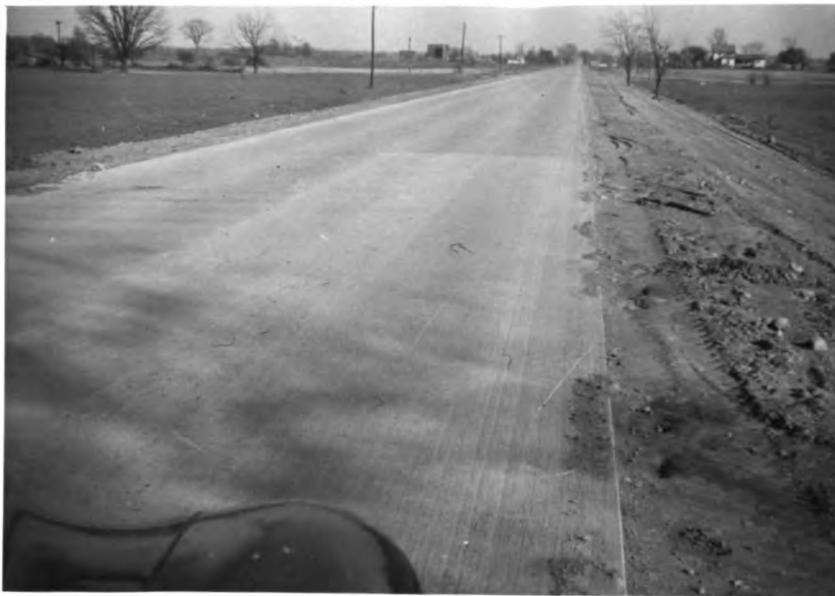
23. General view showing condition of pavement two months after application of white and clear membrane compounds. (11-13-46)
