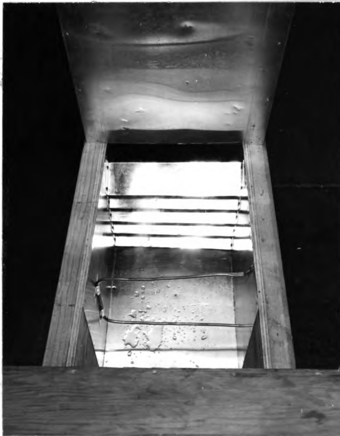
Figure 16. Steam Inlet for Humidifying the Air
