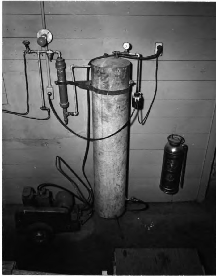
Figure 21. Air Compressor and Supply
