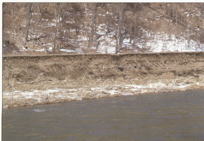
Erosion along ninth hole
