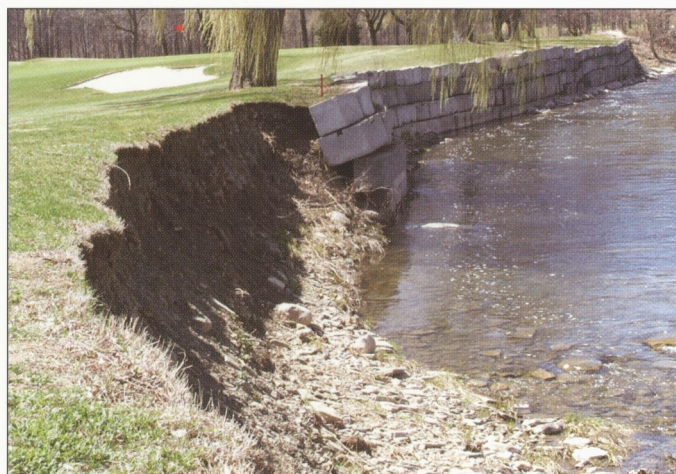
Erosion beside fourth green
