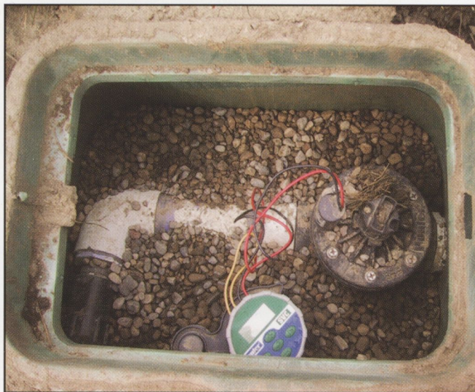
A remote timer has been used to control the electric valve for a zone.
