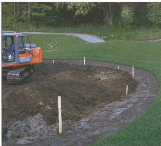
Bad soil conditions on #15 green only compounded the challenge of growing good turf in an already tough area.
