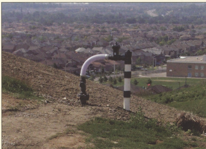
One of the on-site gas wells located to the back of the site. Photo courtesy City of Mississauga
