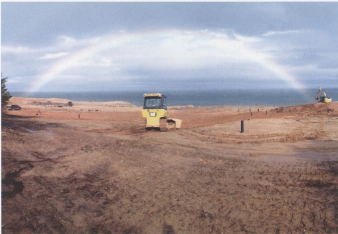
While shaping the 11th fairway it appears the excavator found a pot of gold.
