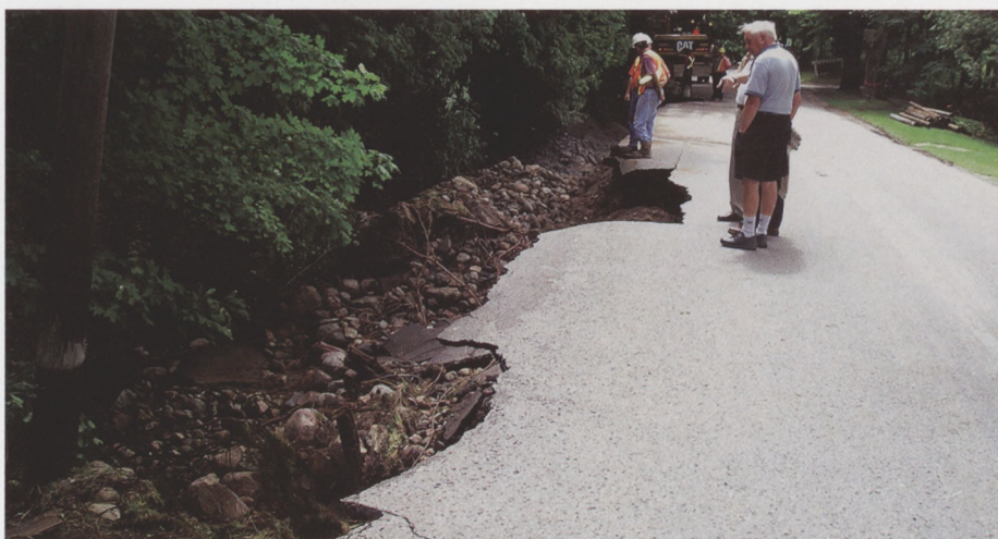
Flood damage at the main entrance drive way, photo courtesy of Kelly Drum.
