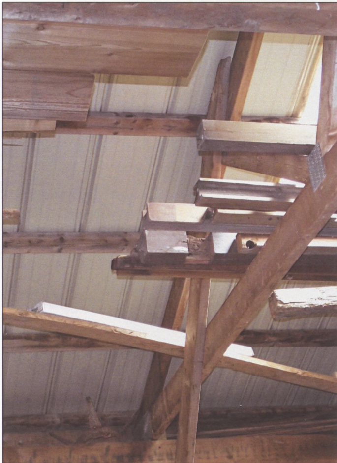
Items that are impossible for workers to safely access.
