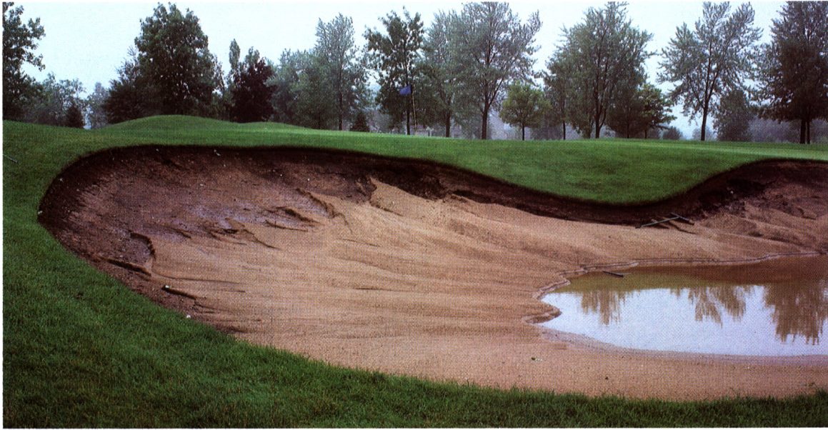
Left: Poor construction or design can lead to serious drainage problems after wet weather and results in more of a penalty than necessary.
