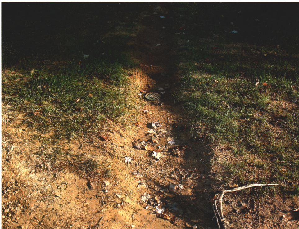
Trench settling will be obvious for years, and therefore trenches need to be properly compacted during installation.
