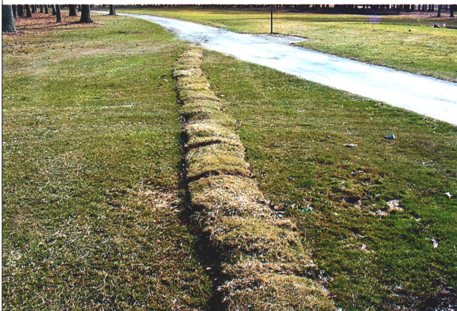
Just mounding the trenches and waiting for settling is not the proper installation technique. New and existing grades should be evenly matched.
