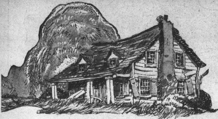
This house is a crumbling ruin from lack of paint. Where paint is not used, deterioration is rapid.
