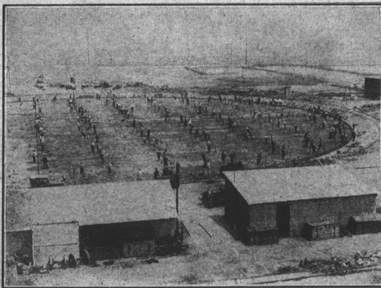
Two hundred and eighty men labored with 250 jacks for five hours, at Long Beach, California, to lower this huge foundation for a municipal gas tank which weighed 370 tons.
