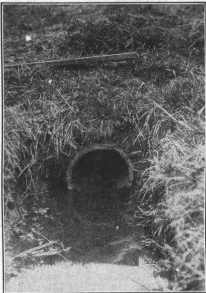
A Poor Outlet for a Tile Drain.
