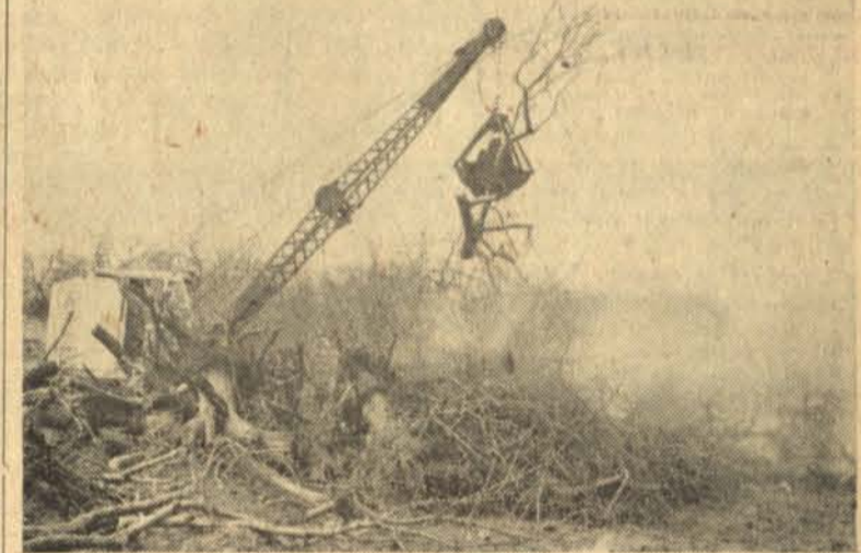
A CRANE and a clam-shell bucket were very handy when it came to piling and burning the downed trees.
