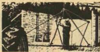
Concrete wall panels are cast flat. Two men and a tractor can raise hardened panels into place in minutes.
