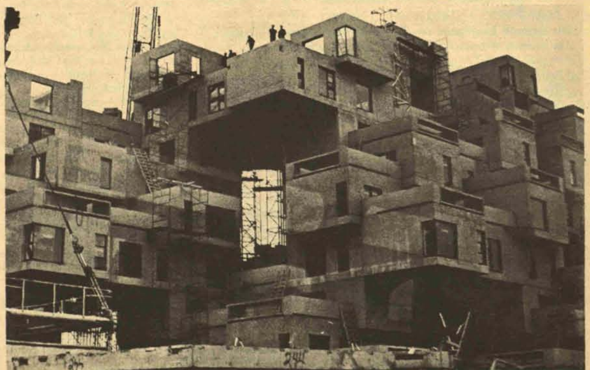
"HABITAT '67" — an unusual concept in multiple city dwellings is an attractive feature of Expo 67. Each of the 158 apartments in this 7-story complex has its own garden on the roof of the unit below. Interconnected walks allow easy access and a community social life. Units were pre-cast and lifted into position. 36 furnished homes will be open to exposition visitors.
