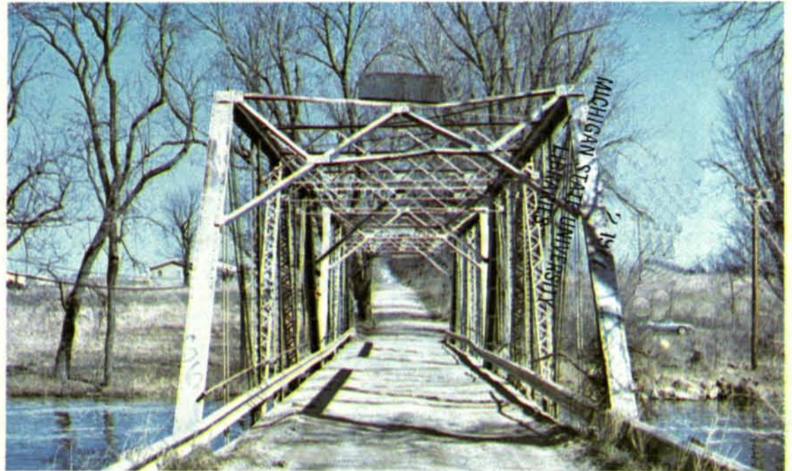
"Load Limit 4 Tons" reads the warning sign before this 1897 bridge on one of Michigan's secondary county roads. 3,721 road bridges in the state have been declared inadequate by county road commissions. 50,475 miles of roads have also been placed in this category. With limited revenue in the Motor Vehicle Fund for road improvement, attempts are being made to divert these funds for other transportation uses.
