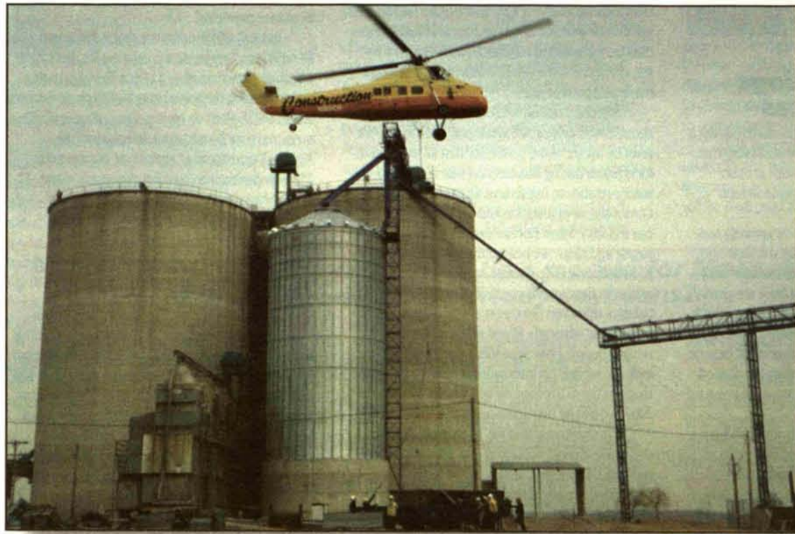
Construction Helicopters, Inc., based out of Ypsilanti, Mich. made quick work in lifting two new grain cleaners, in 6-foot sections, to the top of the Grand Ledge Agri-Sales facility. The Sikorsky S58-T is capable of lifting a maximum of 5,000 pounds. The newly installed cleaners, custom built by Johnson System Inc., are each rated at 15,000 bushels per hour, and will be added to the company's product line and services.
