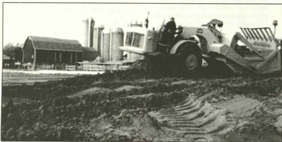
The final rules for EQIP will cost-share up to 75 percent of the cost of certain conservation practices, such as construction of manure management facilities.
