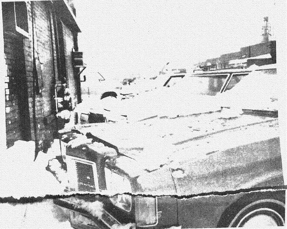
FALLING ICE: No one was injured last Wednesday when a heavy accumulation of snow and ice fell off the roof of the Dutch Kettle restaurant in Pigeon onto five cars. An estimated $10,000 in damages were reported. DEB McBRIDE PHOTO
