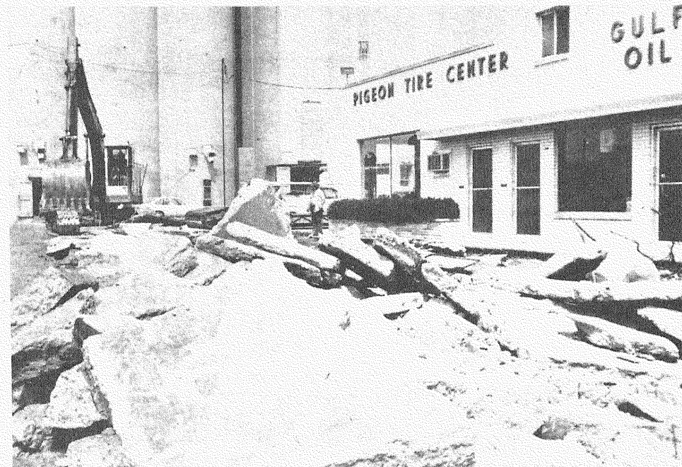
PASSERSBY AT THE CO-OP ELEVATOR CO., petroleum division, have been used to seeing the concrete all turn up in preparation for installing new gas tanks and pumps.
