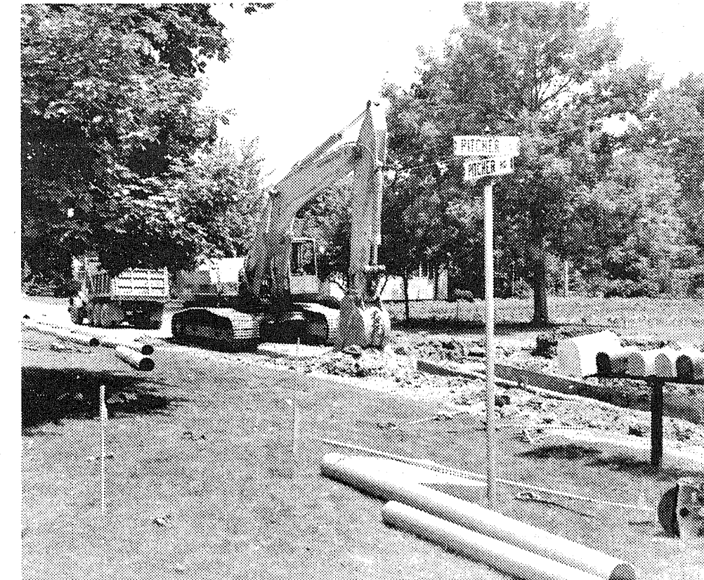
DIGGING IN: As anyone who has driven past the corner of Pitcher Road and Pitcher Court near the new Sebewaing Marina can attest, the work being done there in digging the new Marina basin has changed the local landscape, as this photo shows.
