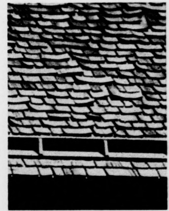
Wood Shingles After Five Years Wear
