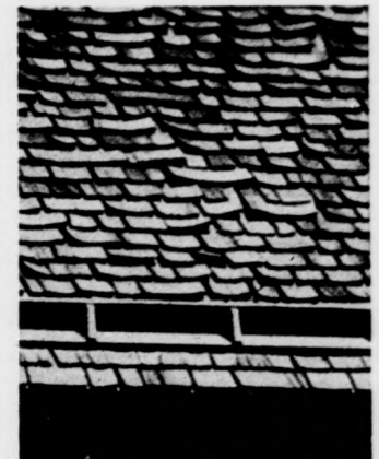
Wood Shingles After Five Years Wear
