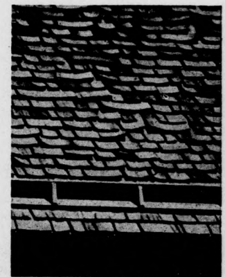
Wood Shingles After Five Years Wear
