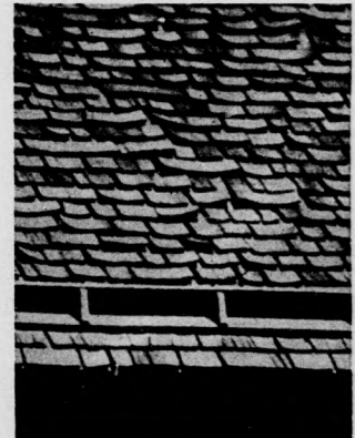
Wood Shingles After Five Years Wear
