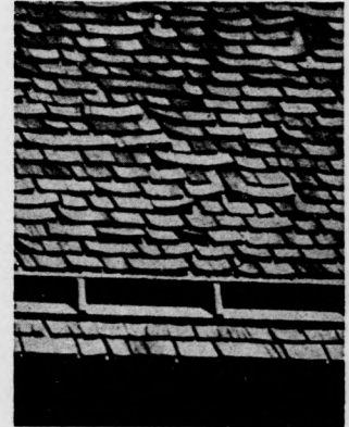
Wood Shingles After Five Years Wear
