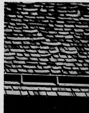
Wood Shingles After Five Years Wear
