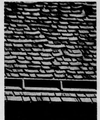
Wood Shingles After Five Years Wear
