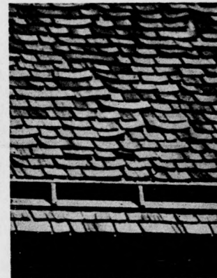
Wood Shingles After Five Years Wear
