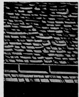
Wood Shingles After Five Years Wear
