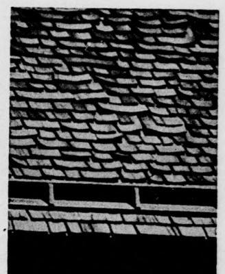
Wood Shingles After Five Years Wear
