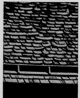
Wood Shingles After Five Years Wear
