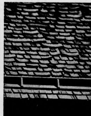
Wood Shingles After Five Years Wear
