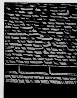
Wood Shingles After Five Years Wear
