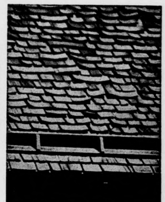
Wood Shingles After Five Years Wear
