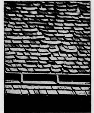
Wood Shingles After Five Years Wear
