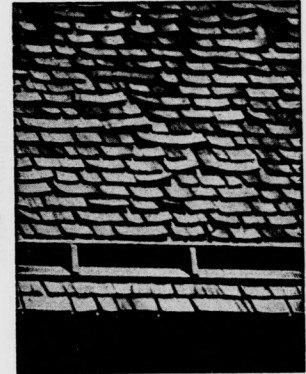
Wood Shingles After Five Years Wear
