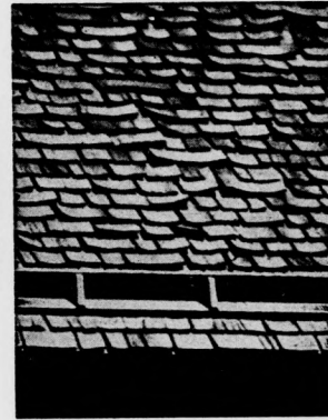
Wood Shingles After Five Years Wear
