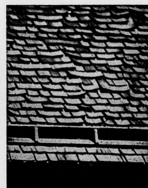
Wood Shingles After Five Years Wear
