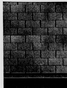
Reynolds Slate Shingles After Five Years Wear
