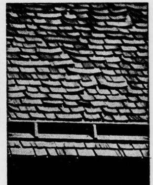
Wood Shingles After Five Years Wear
