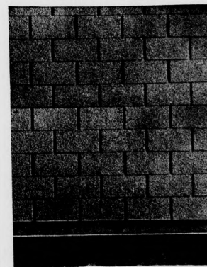
Reynolds Slate Shingles After Five Years Wear
