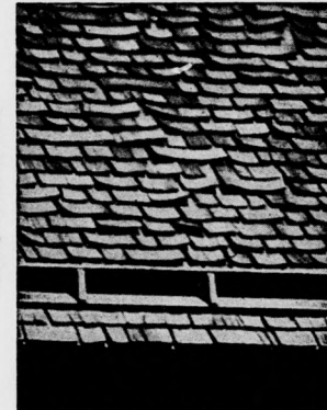
Wood Shingles After Five Years Wear
